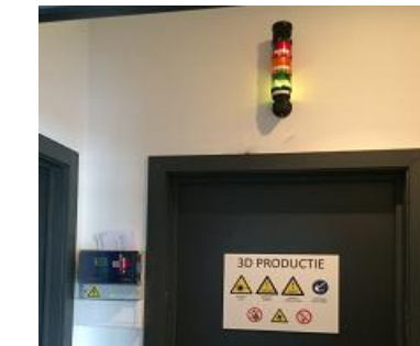
Safety installation at the entrance of a customer lab
